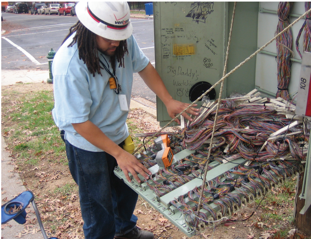
Verizon corrects a cable failure at Eighteenth Street and Trenton Place, SE. The PSC is addressing issues related to the maintenance of the copper (landline) system.
