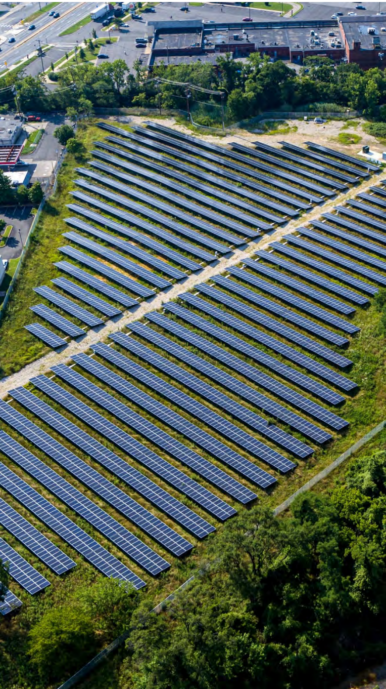
COMMUNITY SOLAR INSTALLATION AT OXON RUN (WARD 8)
